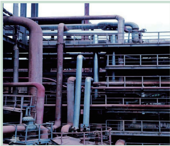
Use of dilution tank and dilution slot for heating process
