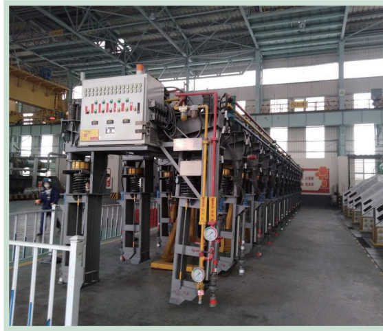
The upgraded busbar lifting frame
